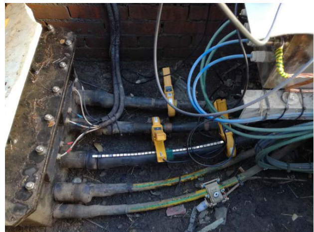
Fig. 5: Sheath current measurements at LB1 of line 1
